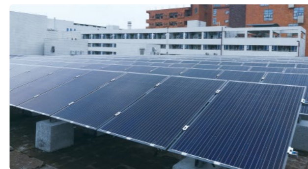
A solar power generating system(Tamron Optical(Foshan)in China)
