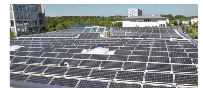
Solar power generation system (improvement at Tamron Europe)
